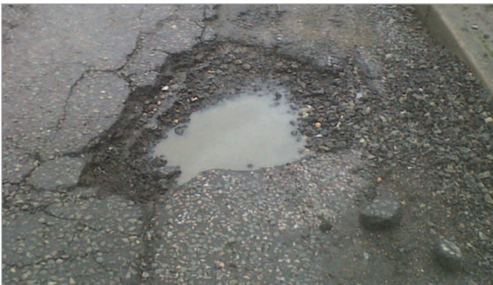
Road damage caused by severe winter weather
