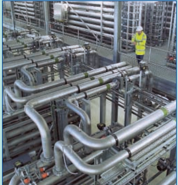
Ultrafiltration Membrane Water Treatment Plant, Three Valleys Water
